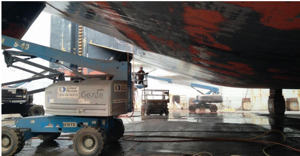
Figure 5: Multiple UHP Man Lifts in Seaspan Caren
